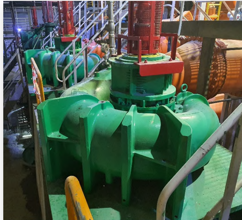
North Bouna Vista, Singapore 6 X L20K pumps
